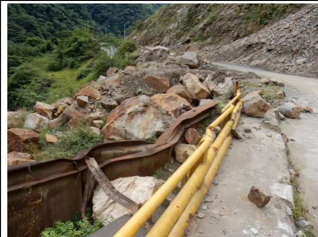
Photo 88: Damages from slope failures along Puerto Valdivia road
