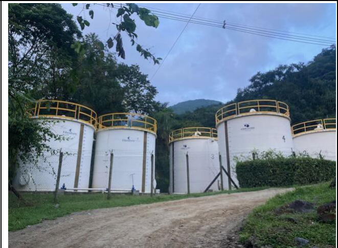
Photo 54: EPM camp potable water storage
