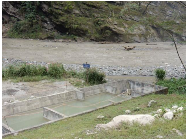
Photo 43: Treatment of drainage water from dam gallery
